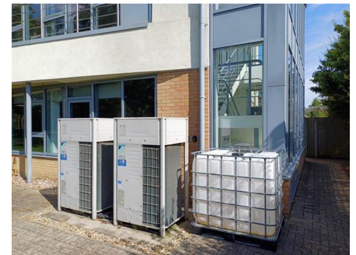
Coppice House Office - Rainwater tank system for watering
